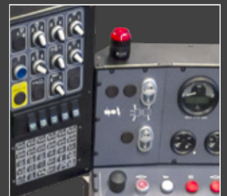
Accurate instrumentation and controls provide a safe and highly realistic training environment
